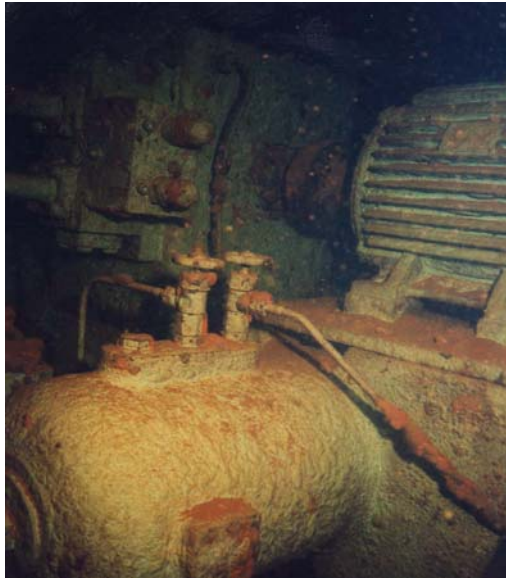
Tales of Deep Penetration in the Engine Room
